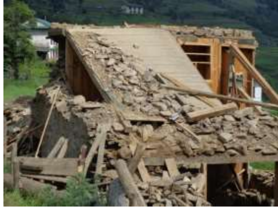
Fully damaged local house of Mapung
