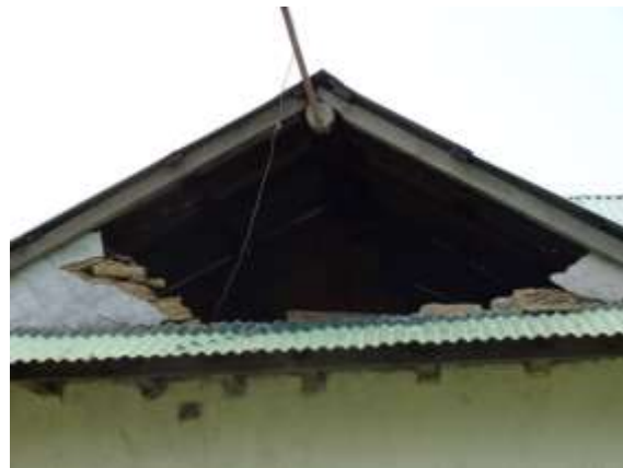
KPHMN – damaged roof
