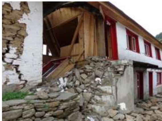
Junbesi School damaged by EQ
